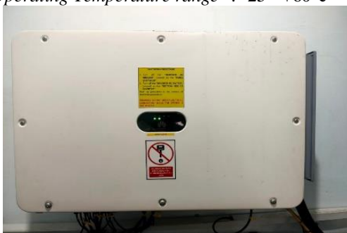
Gambar 6. Inverter 100 KTL di power house
