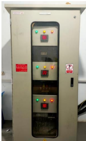
Gambar 8. Panel Box Listrik riset
